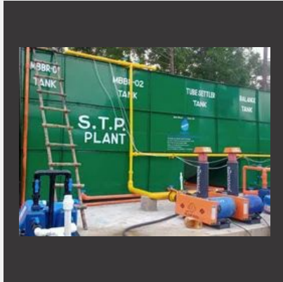
Commercial Sewage Treatment Plant
