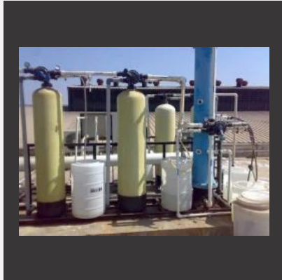
Dm Water Plant
