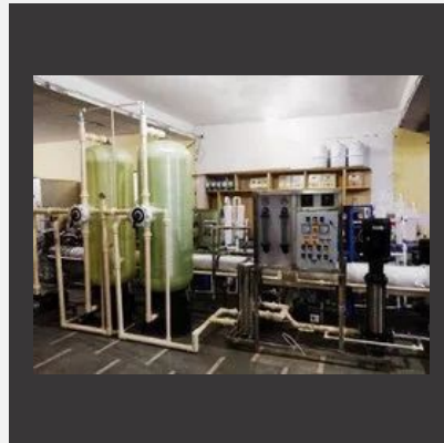
Industrial RO System
