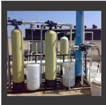
Industrial Dm Water Plant
