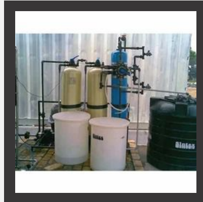
De-Mineralized Water Plant
