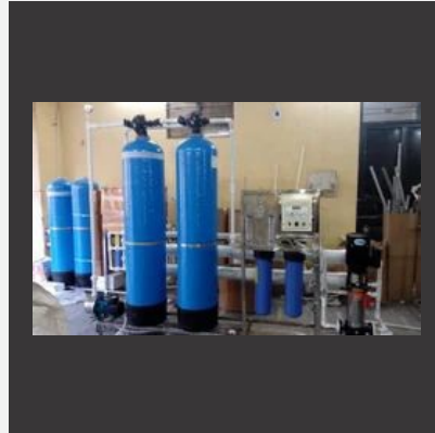
1000 Lph Ro Plant
