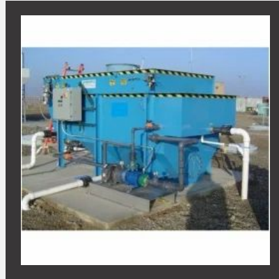
Effluent Treatment Plant
