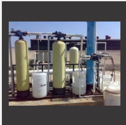
Pure Water RO Plant
